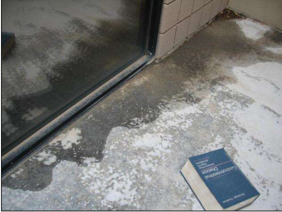
Figure 1: improper slope and water intrusion at master suite balcony has been on going problem.
