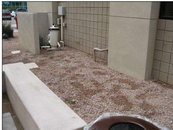
Figure 2: fountain filter system at east end of building
