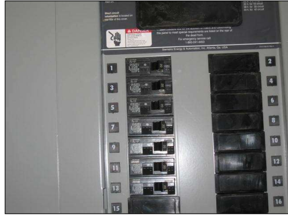
Figure 2: breakers in this panel were showing excessive heat signatures
