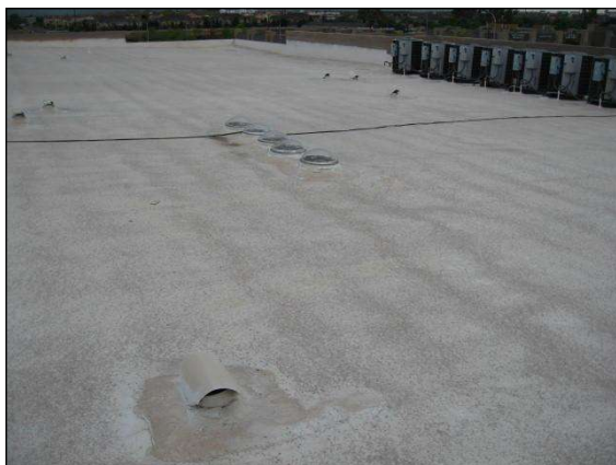
Figure 1: the foam roof has had maintenance done and needs to continue.
