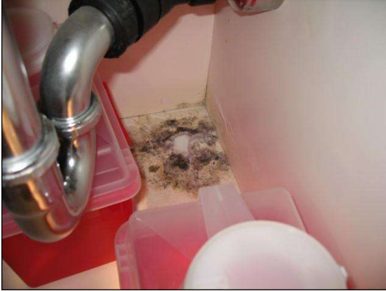
Figure 1: mold/ mildew neds to be cleaned up
