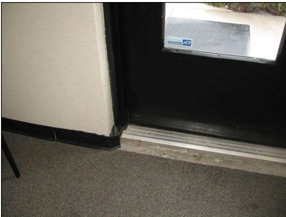
Figure 1: door binds at threshold and needs frame repaired.
