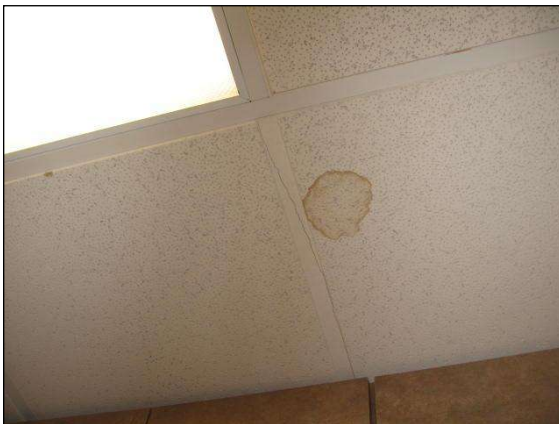
Figure 1: water stains at first floor (a/c line leak?)
