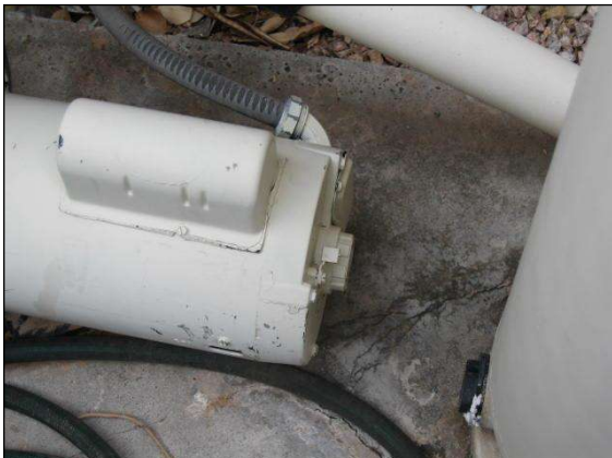
Figure 1: fountain motor missing safety bond
