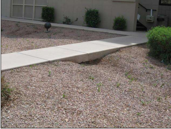
Figure 1: drain not working
