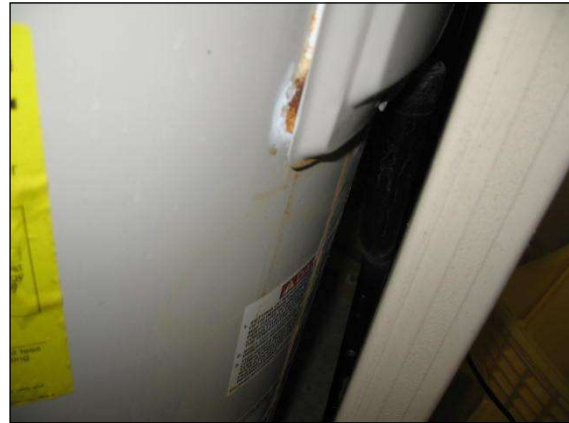
Figure 2: same unit as above at second floor suite and needs replacement.(before damage to other offices from water leaks)
