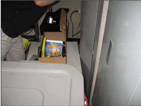
Figure 1: sub panels blocked for access at utility room/ fire safety
