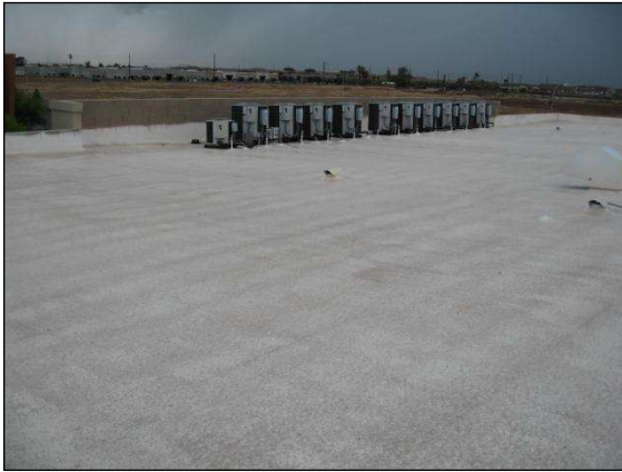
Figure 1: the cmu blocks to the left of the compressors are not capped/ flashed.
