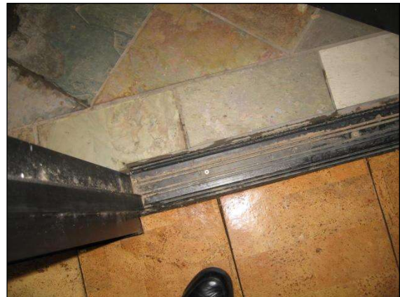
Figure 2: moisture was flowing through threshold plate prior to mopping
