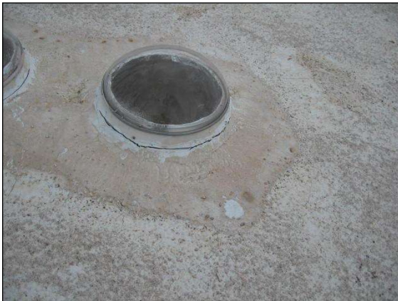
Figure 1: open seams at sky lights need repair
