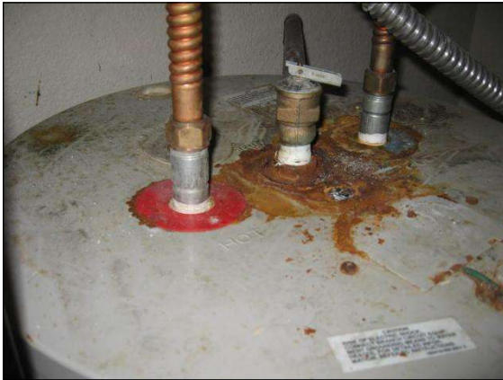
Figure 1: unit at end of useful life corroded at tank body
