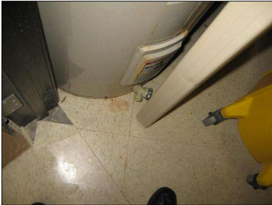
Figure 1: water heaters in all the suites lack a catch pan with a pipe draining to the floor drain
