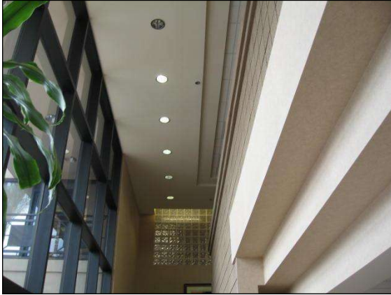
Figure 1: entry lobby ( note light not working)
