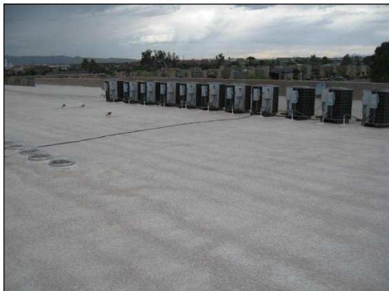
Figure 1: eleven of the 22 units mounted on the roof (facing north)
