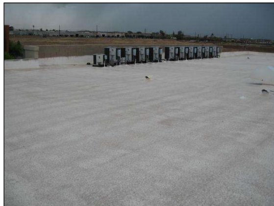
Figure 2: the southside compressors (lighting was flashing in back ground)
