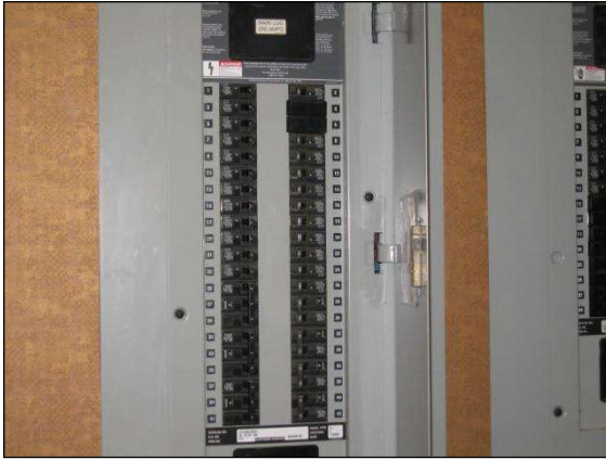
Figure 1: over heated breakers needing maintenance( need system checked for loose connections)
